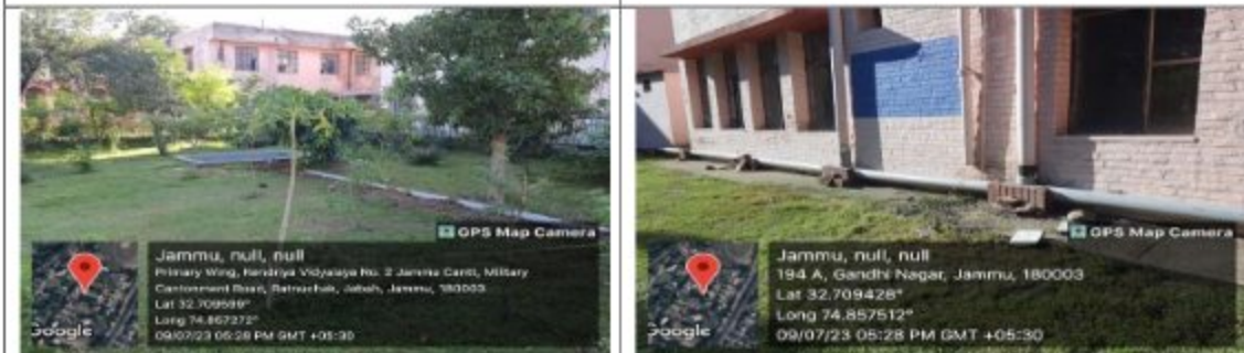
O3. Rainwater collecting pipe and tank
